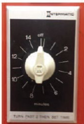
Mechanical Timer Switch Override (Outside the Room)
