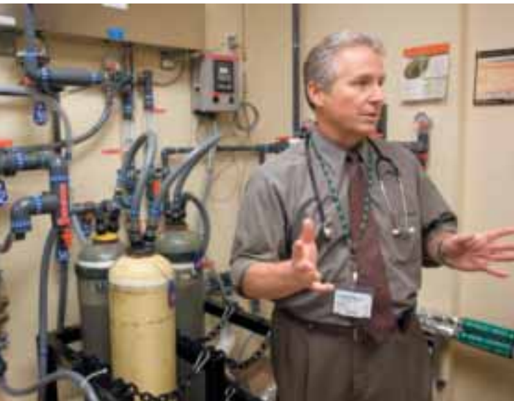
Alexander with the new unit’s water filtration system.
