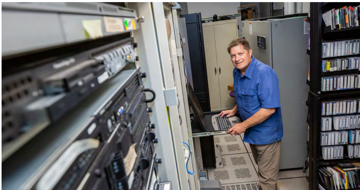
Lee Kozar in a CSBF server room.
